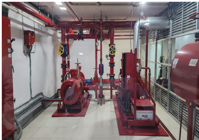
Fire Pump Room
