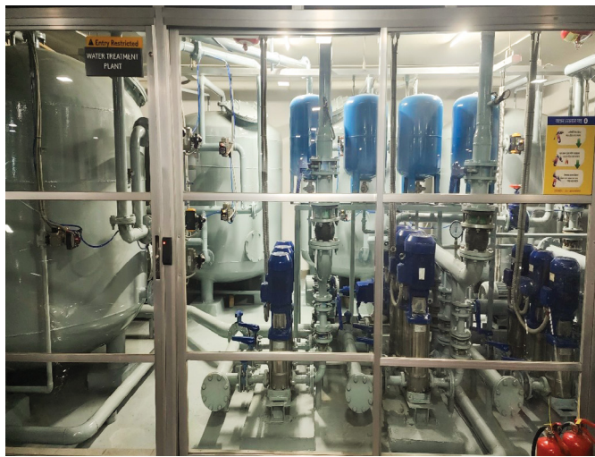
Water Treatment Plant
