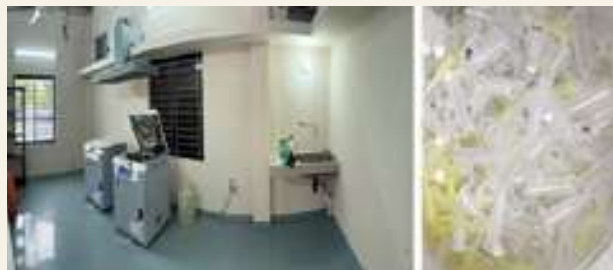
Established waste autoclave facility (Left); waste converted to asset after sterilization (Right)
